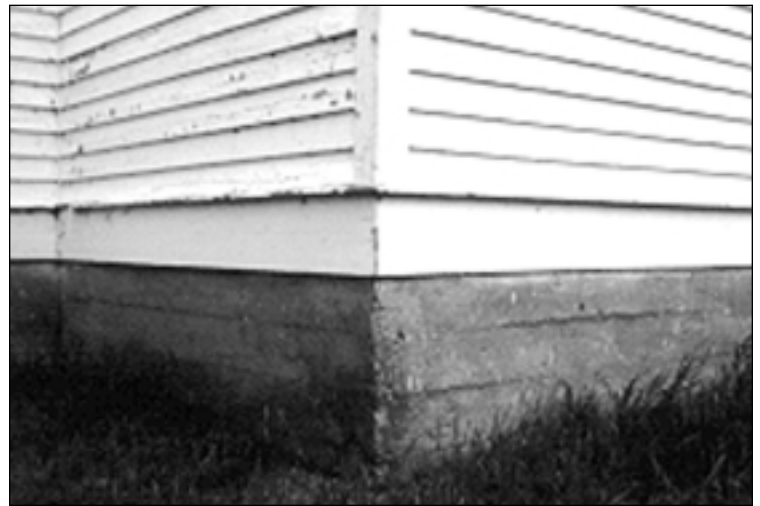
This is an example of a poured concrete foundation, in a church built around 1910.
