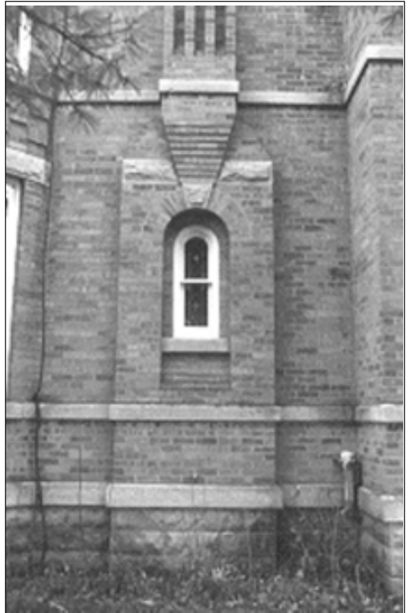
This wall of the J. Engesser House in St. Peter, built in 1888, is a good illustration of the kind of variety in design of which brick is capable.
