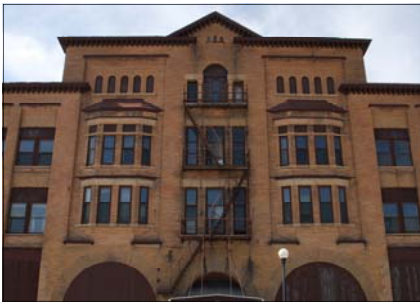
Wayne Hotel, Crookston Vacant since 1996 Tax forfeited property now owned by the County, awaiting rehab at estimated $4 million cost; estimated demolition costs, $500,000
