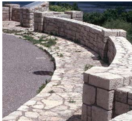
Stillwater Overlook's exceptional design quality makes it an outstanding example of wayside rests erected during the formative years of the state highway department's Roadside Development Division. Built of limestone salvaged from the nearby Minnesota Territorial Prison, the overlook is one of the most elaborate designs by prominent Minnesota landscape architect Arthur R. Nichols (1880-1970).
