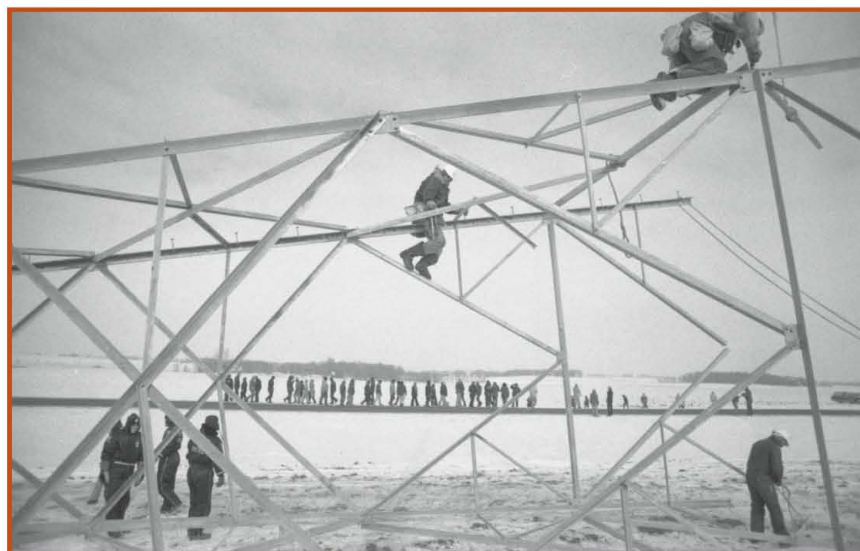
Construction crews assembled a tower while protesters marched in the background near Lowry, MN, February 17, 1978
