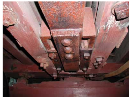
Figure 15: Tannic acid/resin treatment results on metal components with paint remnants.
