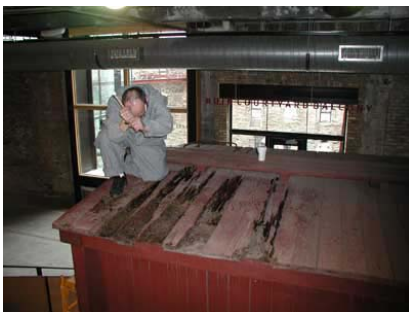
Figure 10: Detail of roof board stabilization in progress. The darker areas show where the liquid epoxy was used.
