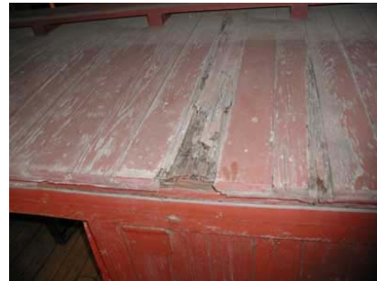
Figure 9: View of deteriorated roof boards before treatment.
