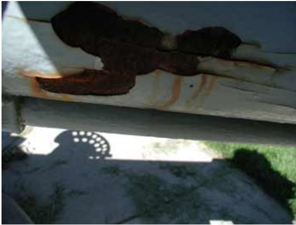
Figure 2. Failed paint and rusting on underside of the barrel.
