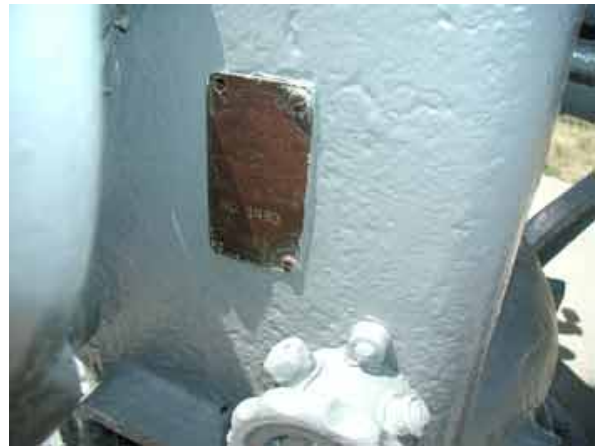
Figure 22. The manufacturer's tag on the PL swivel mount during treatment showing left side screws missing.
