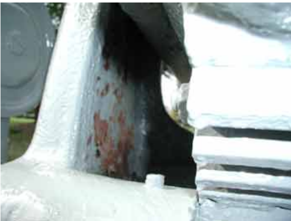
Figure 11. Underside of the swivel mount showing paint loss and corrosion.
